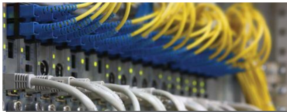
Fibre Optic cables
